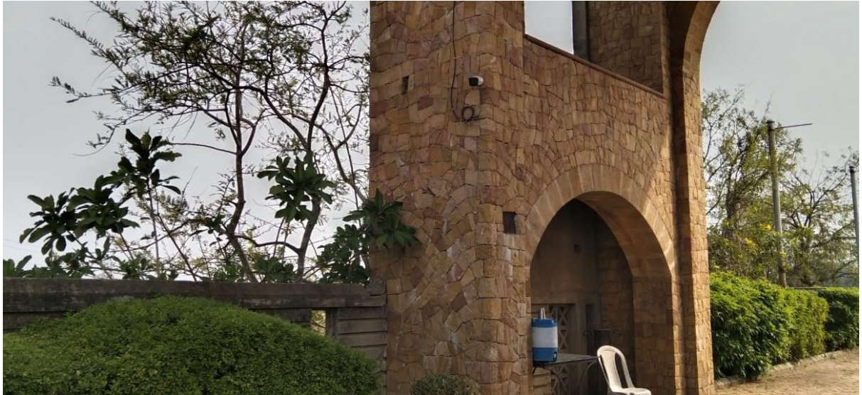
'CCTV Cameras at Entrance'
