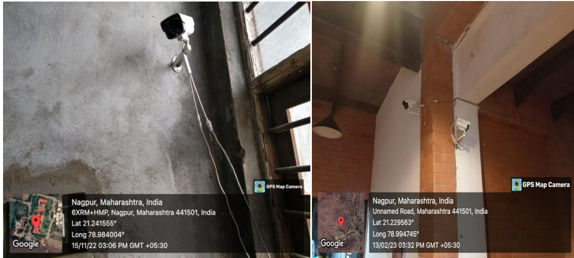
'CCTV Cameras at Corridors'
