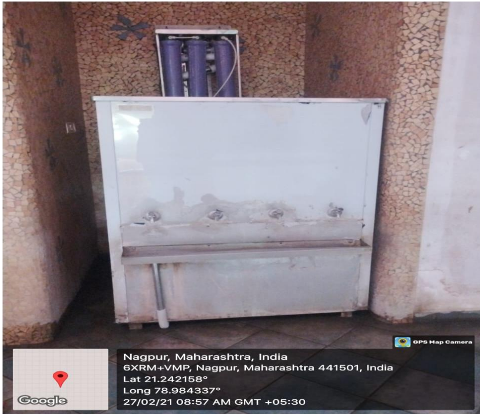
RO Filters installed near water coolers
